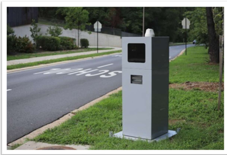
Figure 26 Fixed speed safety camera installed in school zone 12
