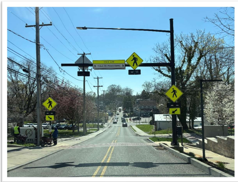
Figure 35 Rectangular Rapid Flashing Beacon (RRFB) 29
